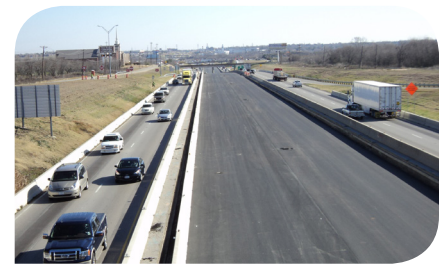
Like the SH 288 Toll Lanes Project, North Tarrant Express Segments 1 and 2 has included extensive work in the median. Our team safely executed the work while minimizing traffic impacts in this dense urban environment.
