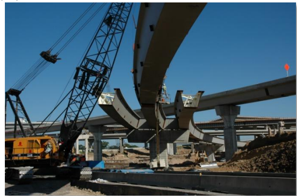
The Katy Freeway Reconstruction Program – was the largest freeway reconstruction program ever performed in the State of Texas and stands as one of the Houston District's most successful projects resulting in the complete reconstruction of twenty-five miles of one of Houston's busiest freeways. All segments were opened to traffic ahead of schedule.
