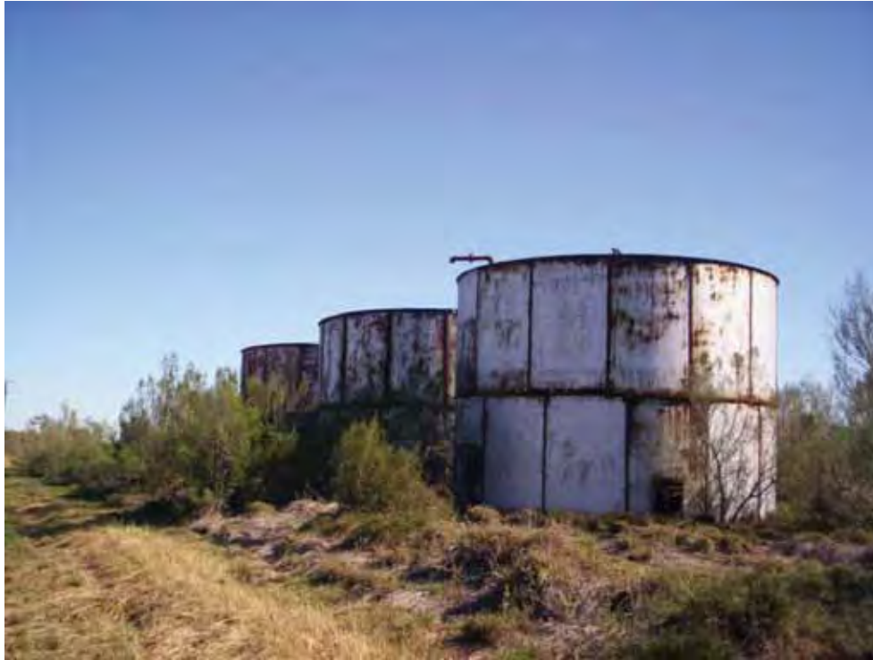
Photo 17 Abandoned tank battery (Map ID 8 – Figure A.4.13-2) with empty ASTs within proposed ROW (December 2008).
