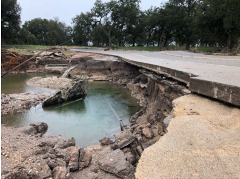
Scour on downstream side of approach due to an overtopping event.
