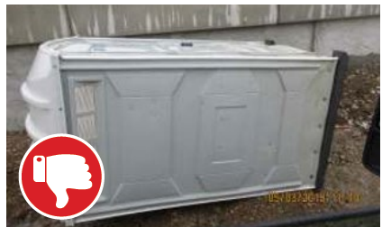
Portable toilet was improperly anchored and has fallen over. Ensure any spills of waste and chemicals are properly addressed.
