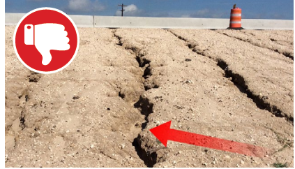
Failing BMP – stormwater is causing the formation of gullies because vegetation stabilization measures were not properly implemented. Stabilize with bonded fiber matrix or erosion control blankets.
