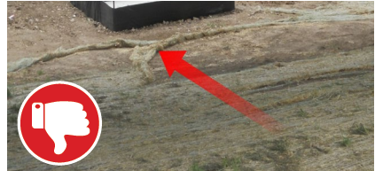
Failing BMP – blanket has begun to degrade and is pulling off of the soil. Replace or re-anchor loosened blankets.
