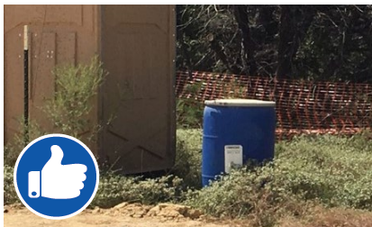
Properly anchored portable toilet in safe, flat location away from storm sewers and drainages.
