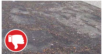
Failing BMP – mulch is generally not appropriate in areas of concentrated flow. Mulch needs to be applied regularly in high traffic areas and should be applied evenly and uniformly and at an appropriate thickness.
