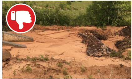
Failing BMP – dam is filled to capacity and in need of maintenance. The check dam should cover the entire length of the drainage. Silt and debris should be removed from the dam on a regular basis.
