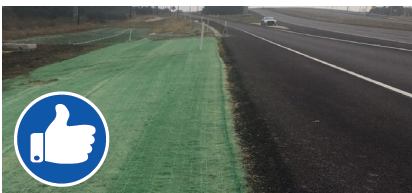
Properly installed blankets – installed below the pavement edge and covers entire area.
