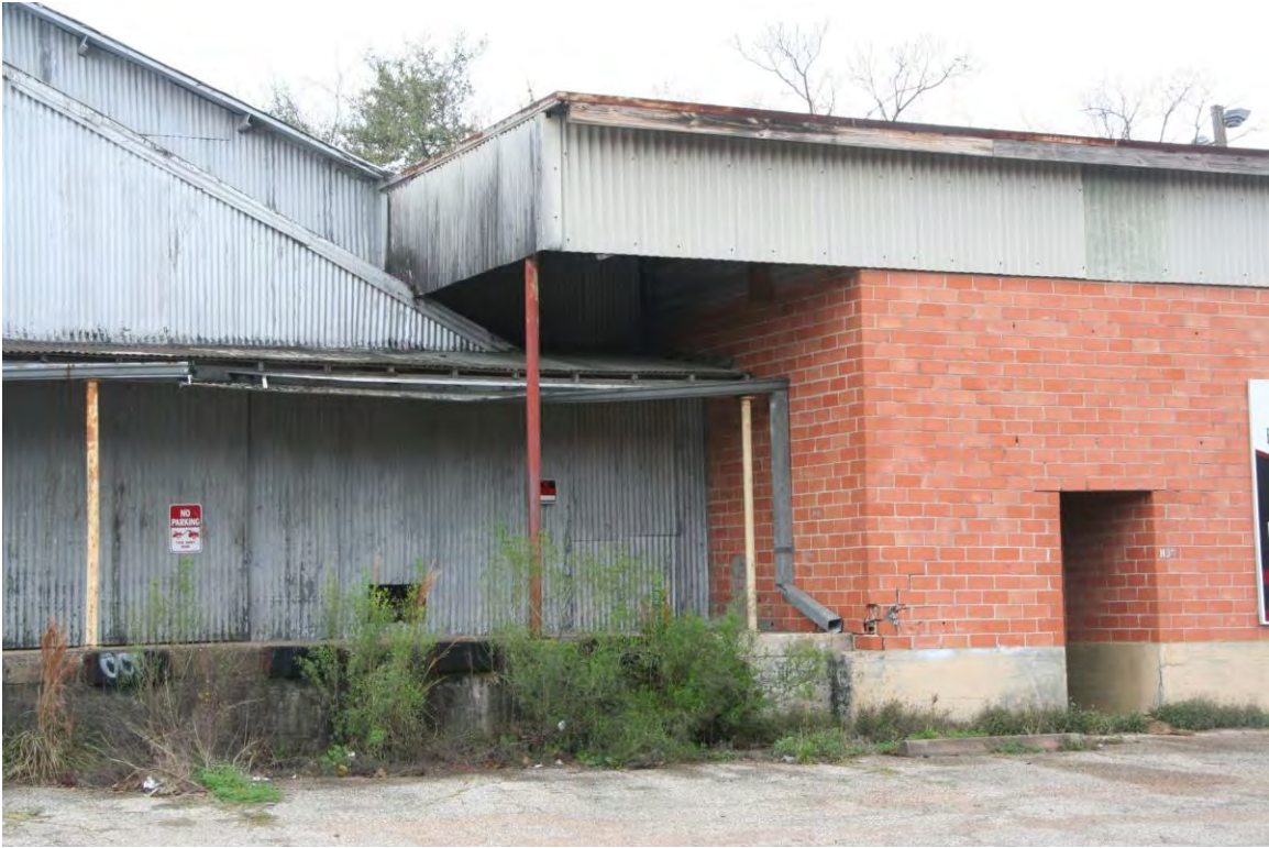
View facing northeast, showing connection between Carlisle Plastic North Warehouse and South Warehouse.
