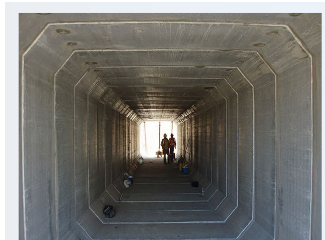
Replacing small old drainage pipes under the freeway with 12'x12' box culverts will greatly increase the capacity to hold stormwater underground and off the streets.
