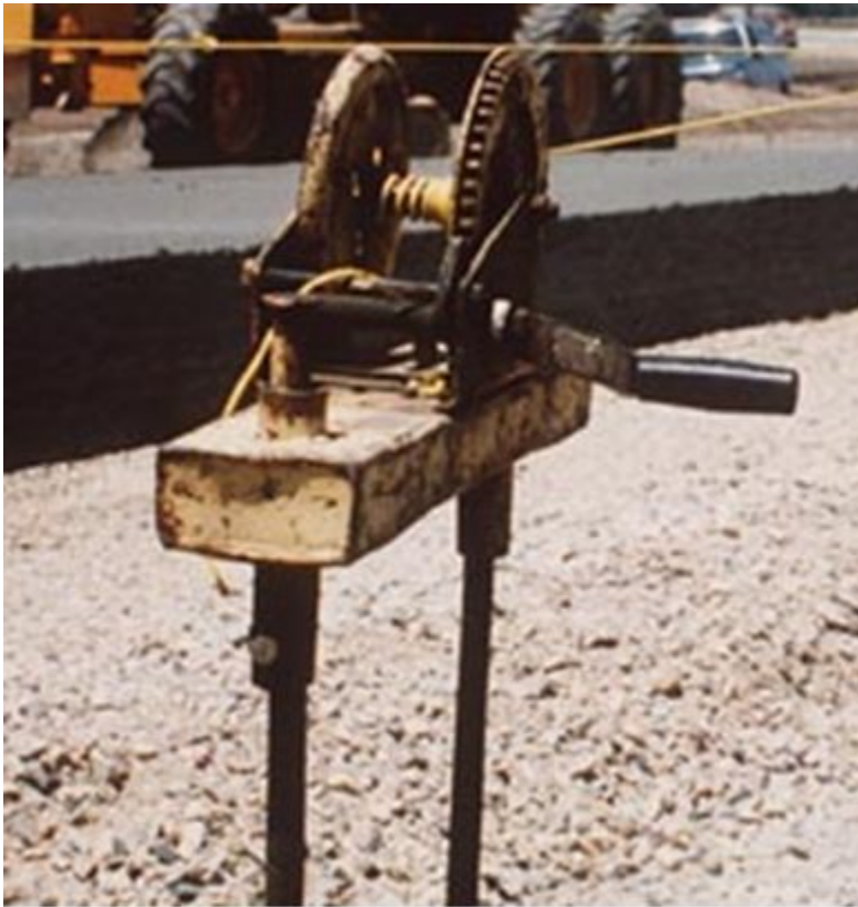
Figure 9-40. Another view of guide wire controls.
