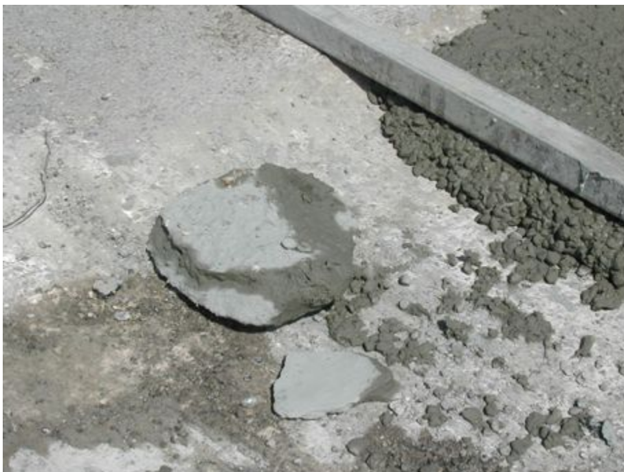
Figure 9-13. Large clumps of concrete.
