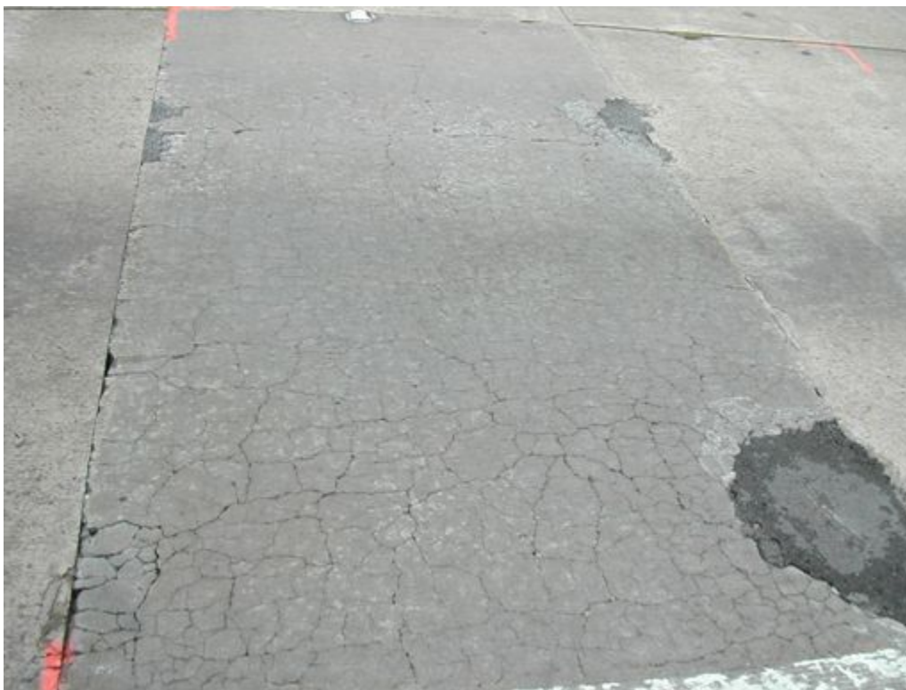
Figure 10-7. Map cracking in FDR slab.
