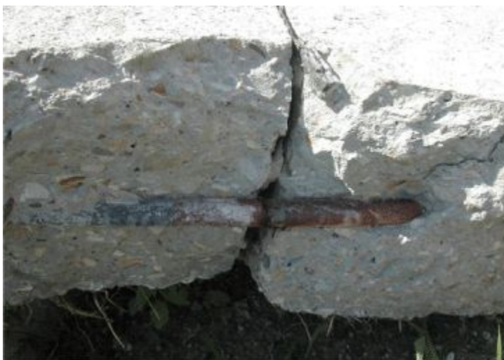
Figure 10-25. Rusted dowel bar.
