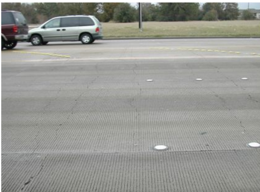
Figure 9-68. Random cracks in CRCP.
