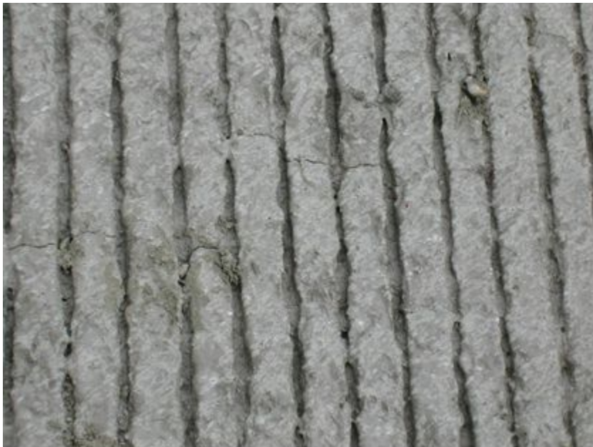
Figure 9-66. Plastic shrinkage cracks.
