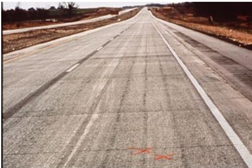
Figure 9-48. Unacceptable – vibrator streaks.
