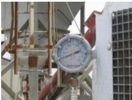
Figure 9-11. Slump meter mounted in the mixing truck.
