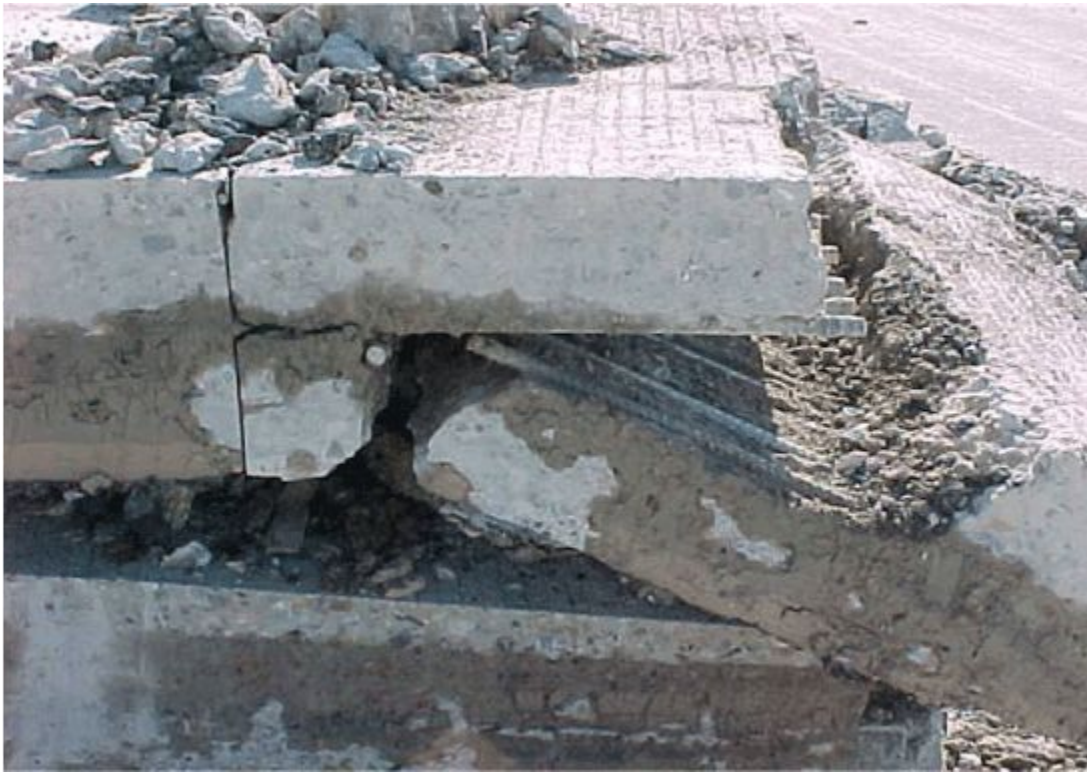
Figure 10-27. Construction joint failure.
