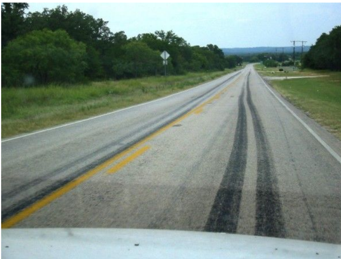
Figure 13-8. Bleeding of seal coats.
