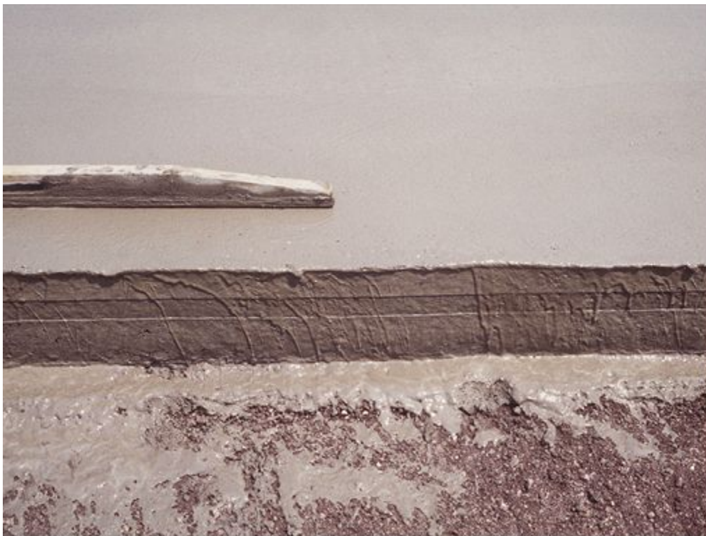
Figure 9-58. Finishing with excessive mortar slurry.
