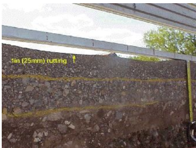
Figure 4-17. Trench sidewalls showing severe rutting.
