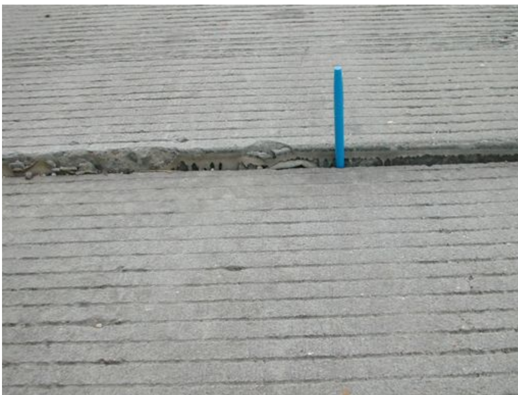
Figure 10-17. Severe faulting at the transverse joint.
