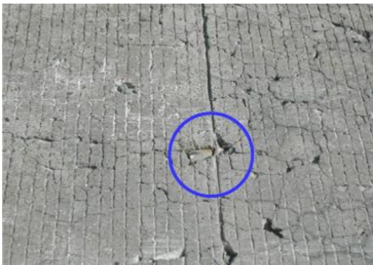
Figure 10-26. Misaligned dowel bar.
