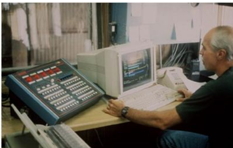
Figure 9-2. Most batch plants are computerized.
